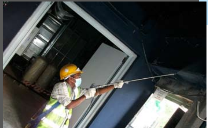
Spray painting machine enables the worker to achieve a smooth finishing while covering a larger area of work in a shorter time.
