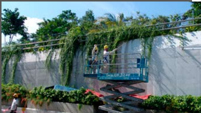
Using a scissor lift removes the need for erecting and disassembling scaffolding as well as cuts down the movement of workers.
